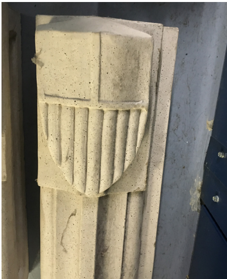
A newly cast replacement for one of the crumbling terracotta pieces from 201's façade.
